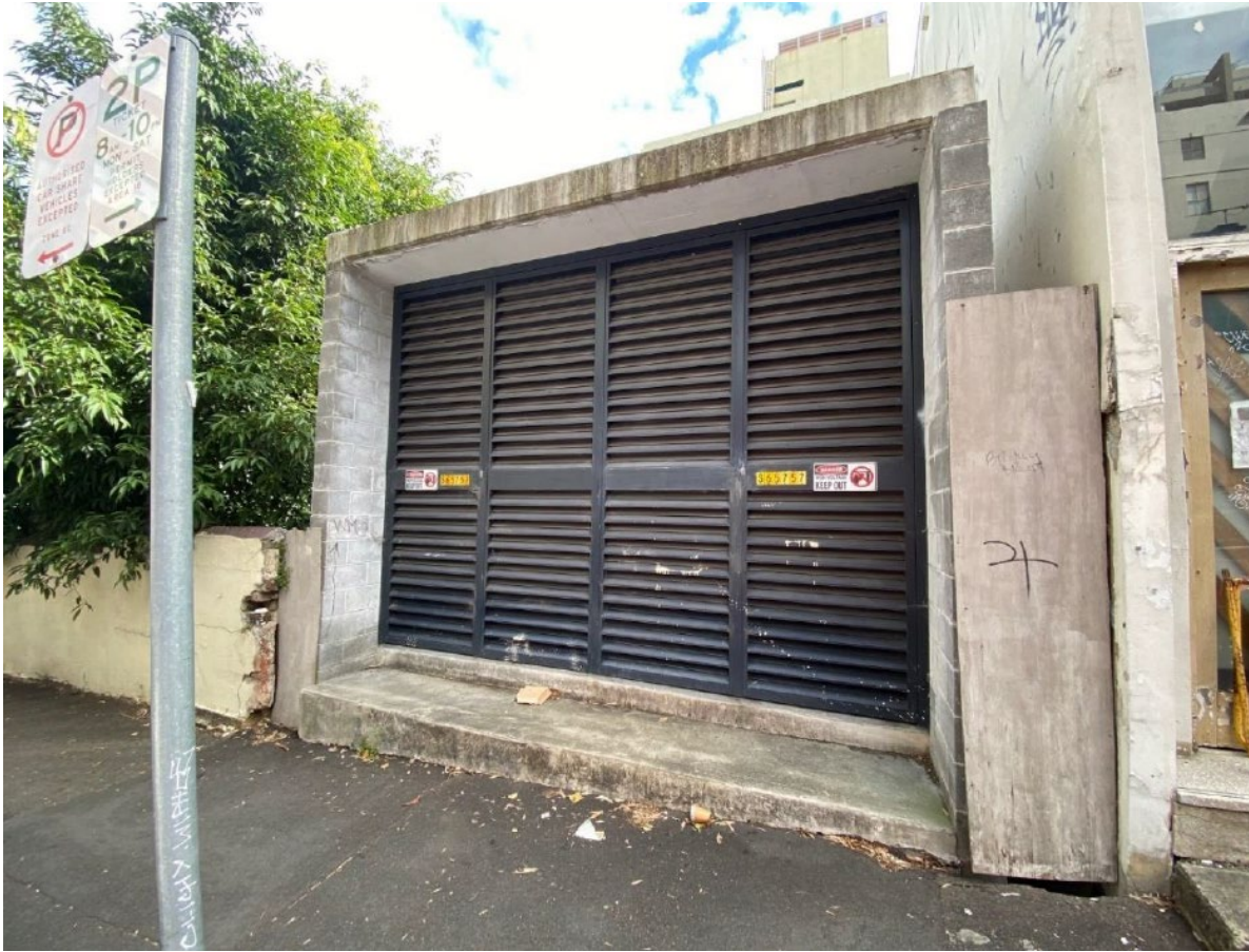
existing substation to be retained on the Commonwealth Street frontage
